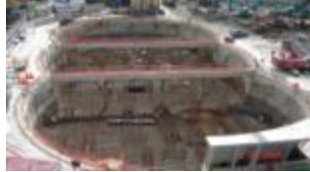
Fig. 1 Peanut shape formed by 30m diameter diaphragm wall panels at The Sail @ Marina Bay
