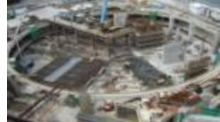
Fig. 2 2 levels of RC circular ring slab and beam (50m diameter each) constructed at SOHO @ Eu Tong Seng Street
