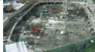
Fig. 8 Tribeca residential project with 2 basements using counterfort diaphragm wall panels and counter slab with perimeter diaphragm wall
