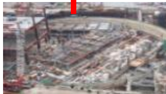
Fig. 5 Marina Bay Sands Integrated Resort South Podium Donut of 120m diameter excavation site
