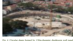
Fig. 4 Circular shape formed by 130m diameter diaphragm wall panels at City Square residential project at Jalan Besar/Kitchener Road
