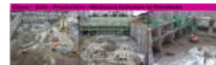
Fig. 15 These are site photos of Strut-Free counterfort diaphragm walls system adopted in South Korea
